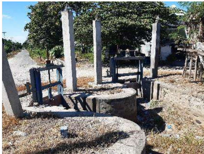
Figure 22. Condition of the Sluice in Langaleso Village
